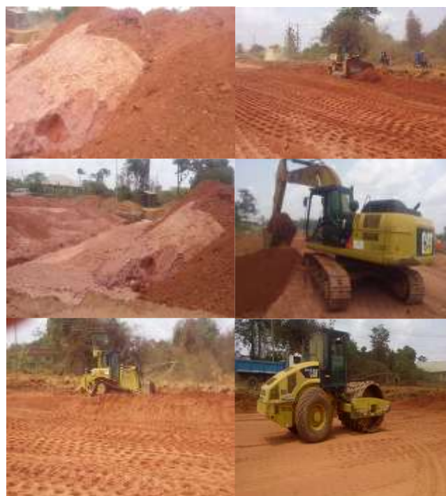
Fig. 3. Some of Site photographs taken along the roadway showing different construction processes and machine/equipment.
